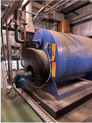
Existing Domestoc HW boiler.
