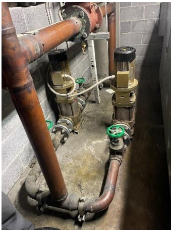
Existing CW. transfer pumps.
